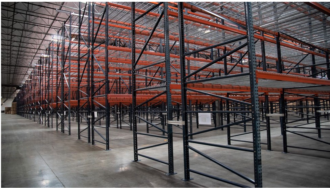
150K SF building, fully racked, designed and permitted for oversized pallets. Highly complex product placement, product classification, complete with emergency egress lighting.
